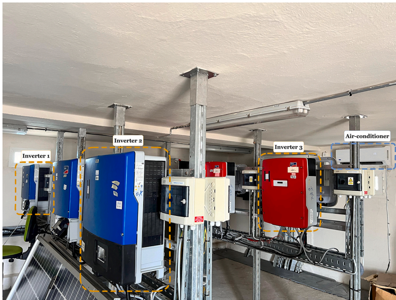
Fig. 23. Inverters in a temperature-controlled environment for optimal performance.
