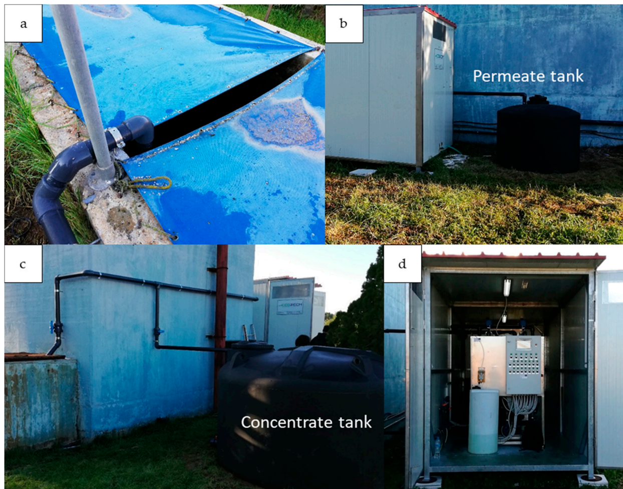
Figure 2. Pilot UF membrane unit installation at Patras' wastewater treatment plant, (a) membrane feed, (b) permeate tank, (c) concentrate tank, and (d) membrane unit housing.
