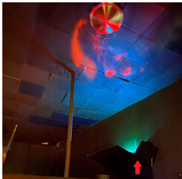
Figure 2. Bare-bulb germicidal ultraviolet lower-lip installation. Ballast with bare bulb affixed to wall with reflecting up-sloping lower-lip underneath to shield occupied space from direct UV-C photons. Limited blue light in the visible spectrum emitted from the fixtures is seen above and a ceiling fan in the foreground. A red arrow points to the location of the hidden bulb behind the up-sloping lower lip.
