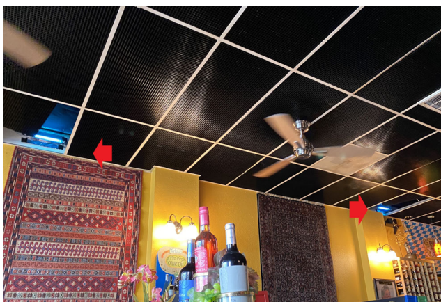
Figure 1. Low-dose upper-room germicidal ultraviolet with eggcrate ceiling. Perforated ceiling tiles are removed to show two of the four 1.6-W output UV-C fixtures. Faint blue light emitted in the visible range from germicidal UV fixtures is seen near-left and far-right and ceiling fan blades are evident. Red arrows point to the bare GUV bulbs above the eggcrate.
