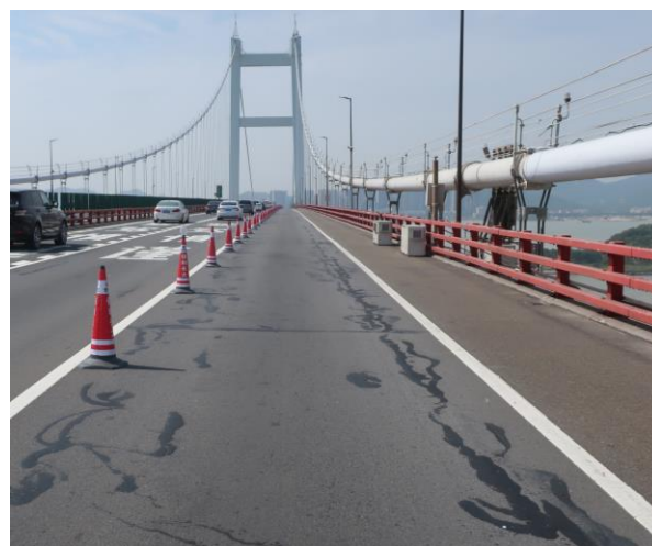
Figure 19. Photograph of fatigue cracking in the steel bridge deck EAC pavement.
