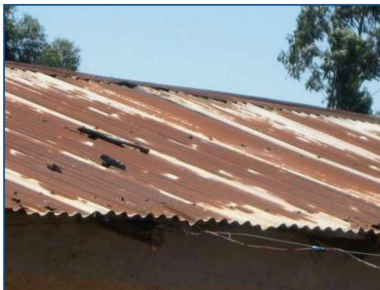
Figure 1 Corrosion on corrugated iron roof sheets close to factory due to air pollutions.
