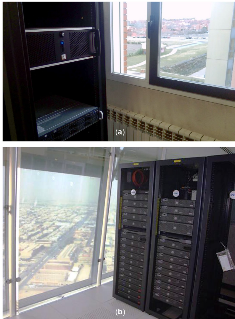
Fig 1. Server racks with a view to the outside. (a) A picture taken at author's (J.C.G.-E.'s) own university. (b) Computer server room in Al-Faisilya Tower, Riyadh, Saudi Arabia [37].
