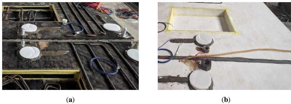
Figure 3. Different types of isolation layers in ballastless tracks. (a) Rubber isolation layer; (b) geotextile isolation layer.
