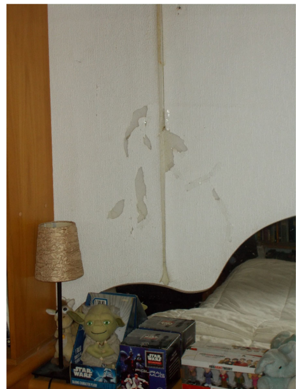
Fig. 3 Dampness on the wall (F.H. 57-year-old man)
