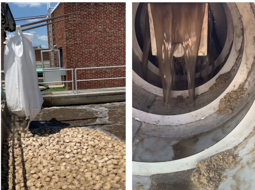
FIGURE 1 (Left) Mobile-biofilm carriers (i.e., kenaf) are compressed and packed in sacks and are easily integrated with an existing WWT process. (Right) Mobile-biofilm carriers are retained by screens, discharged into a sump, and flow with screen wash water into a location selected for their reintroduction to a WWT process.
