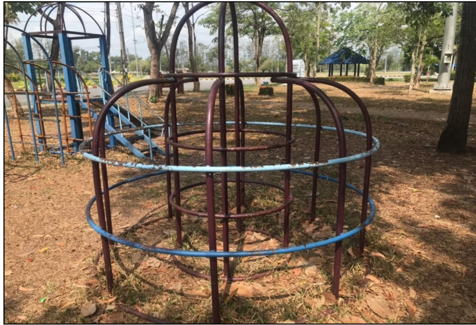
Figure 3. Jungle gym: The height from the floor was more than 1.8 m where a child might fall. There were no safety rails. The distance between the stairs was more than 32 cm. Color paint had peeled off of the playground equipment.
