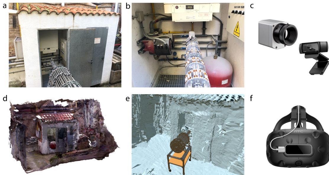
Figure 12. (a) Boiler room with the robot prepared to perform an inspection. (b) First-person view of the robot and the thermal camera located in the end-effector. (c) Two sensors were used in the real environment: an Optrix PI thermal camera and a Logitech RGB camera. (d) On the other hand, the real scenario was reconstructed using a Kinect and the software RTAB-Map. (e) Then, it was imported in Virtual Reality with a model of the robot. (f) The operator uses the HTC Vive VR headset and the Leap Motion controller to teleoperate the real robot from a remote and safe location.
