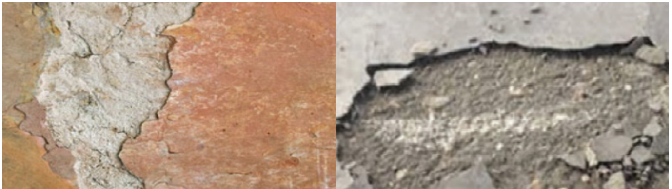
Figure 2. Sample images of concrete with delamination defects.
