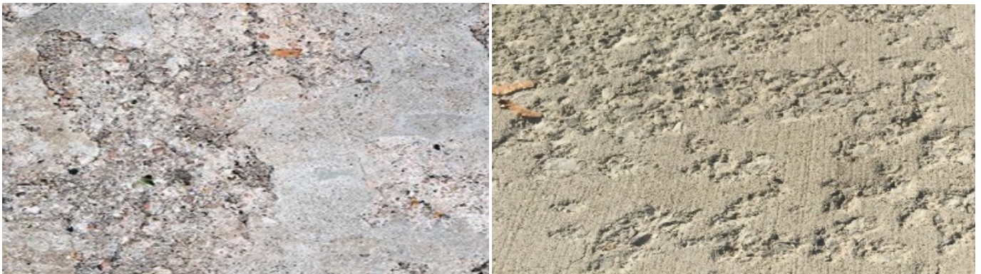
Figure 4. Sample images of concrete with spalling defects.
