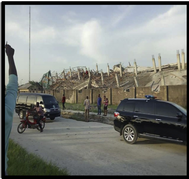
Figure 5. 8-storey hotel building after collapse in Owerri Metropolis Imo State. Source: Author (2020).
