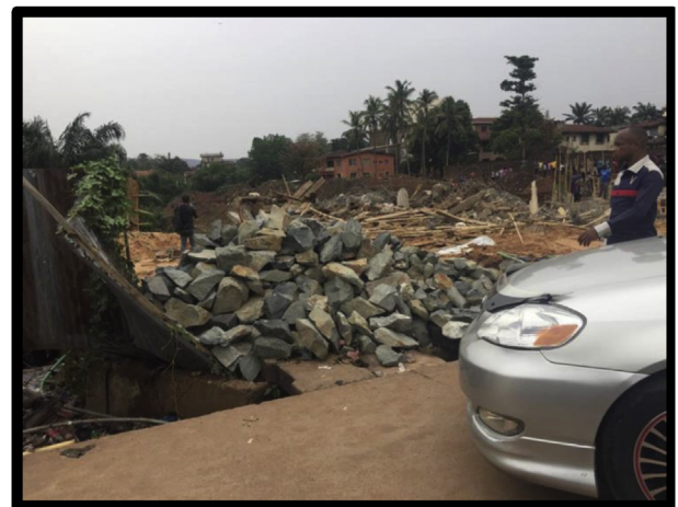
Figure 10. The debris of collapsed site along O'connor Street, Enugu. Source: Authors' fieldwork (2020).
