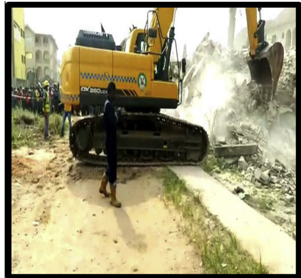
Figure 3. The collapsed building project in under controlled demolition in Lagos State. Source: Authors' (2020).
