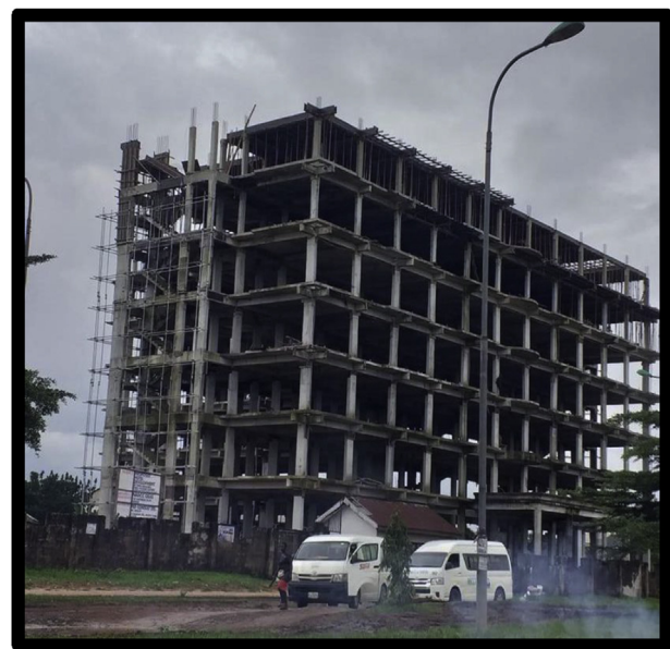
Figure 4. 8-storey hotel building before collapse in Owerri Metropolis Imo State. Source: Author (2020).
