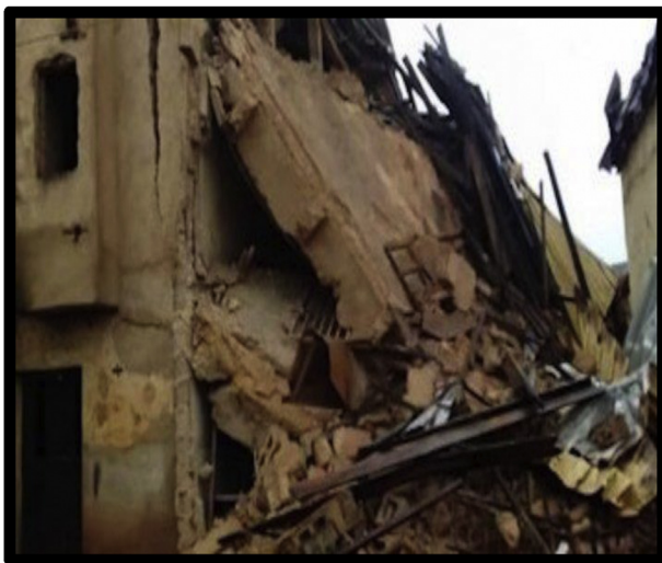
Figure 2. The collapsed building project in under controlled demolition in Lagos State. Source: Authors' (2020).
