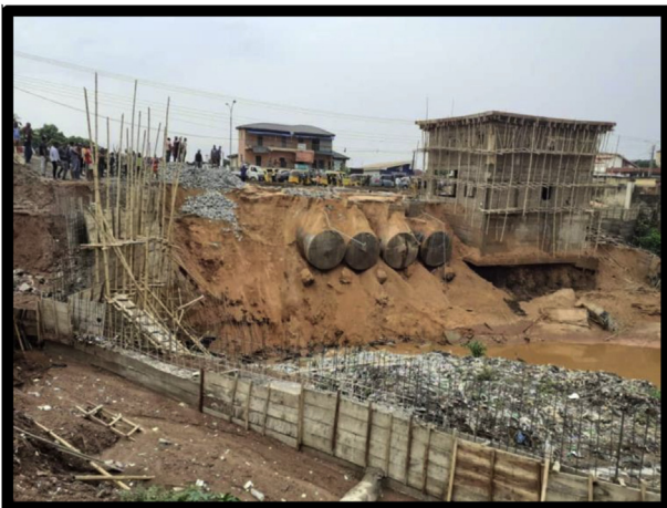
Figure 8. The building project on water ways along O'connor Street, Enugu. Source: Authors' fieldwork (2020).
