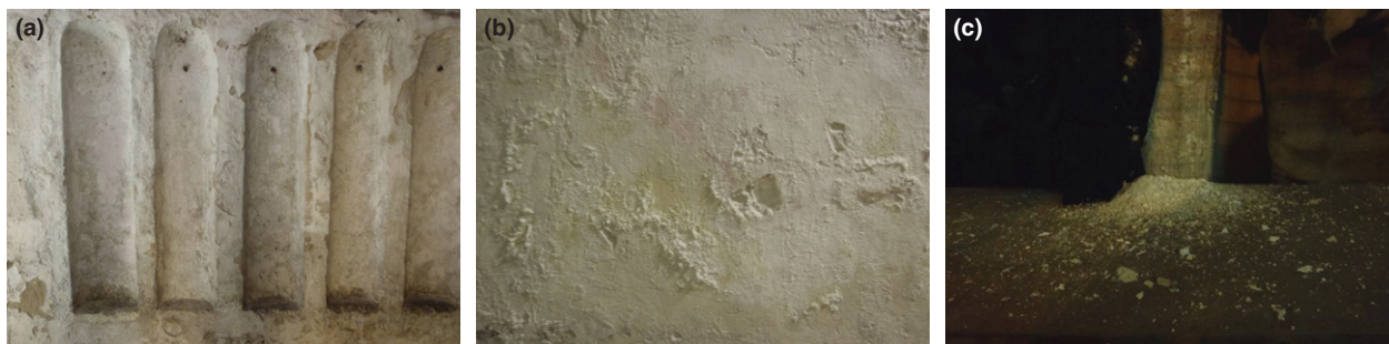
Fig. 2. (a) Pink discoloration of the wall caused by halophilic Bacteria . (b) Salt crusts of sodium chloride on the walls. (c) Detached salt contaminating other materials (pictures: Sterflinger).
