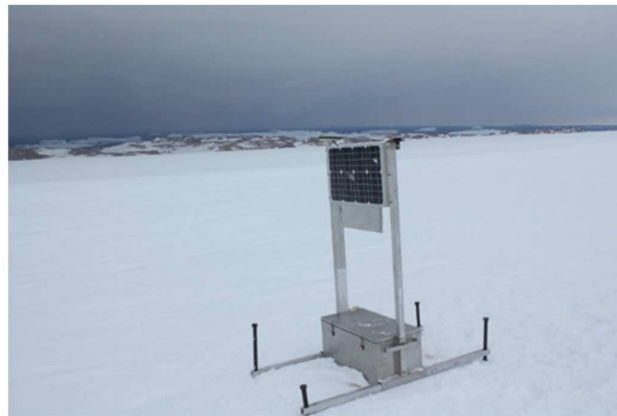
Figure 9. The installation site in Antarctica.
