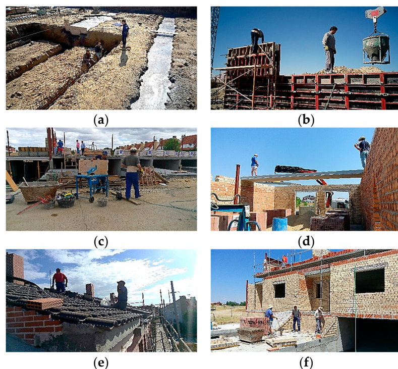
Figure 4. Construction systems during the different execution phases: (a) foundation; (b) reinforced concrete walls; (c) urbanization; (d) precast slabs; (e) roofs; (f) facades.
