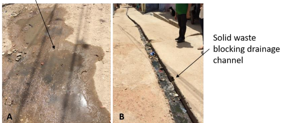
Figure 4. (A,B) Blocked and inadequate drainage, with mosquito larvae in standing water outside dwellings in favelas, Fortaleza, Brazil.
