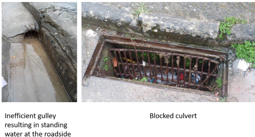
Figure 3. Conventional drainage, Ouro Preto, blocked with solid waste.
