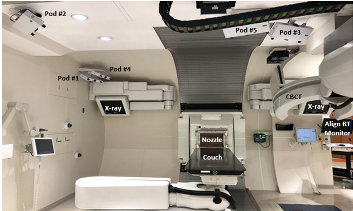
FIGURE 4 The proton half-gantry room with its busy ceiling space after the installation of the 5-camera system
