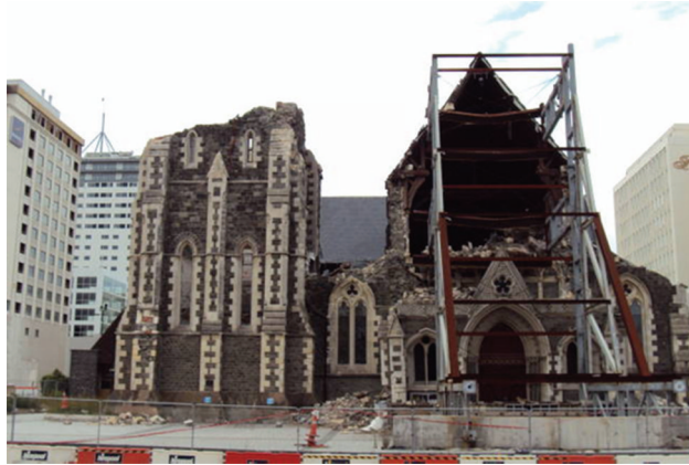
FIGURE 1: The Christchurch cathedral after the February 22, 2011 magnitude 6.3 earthquake.
