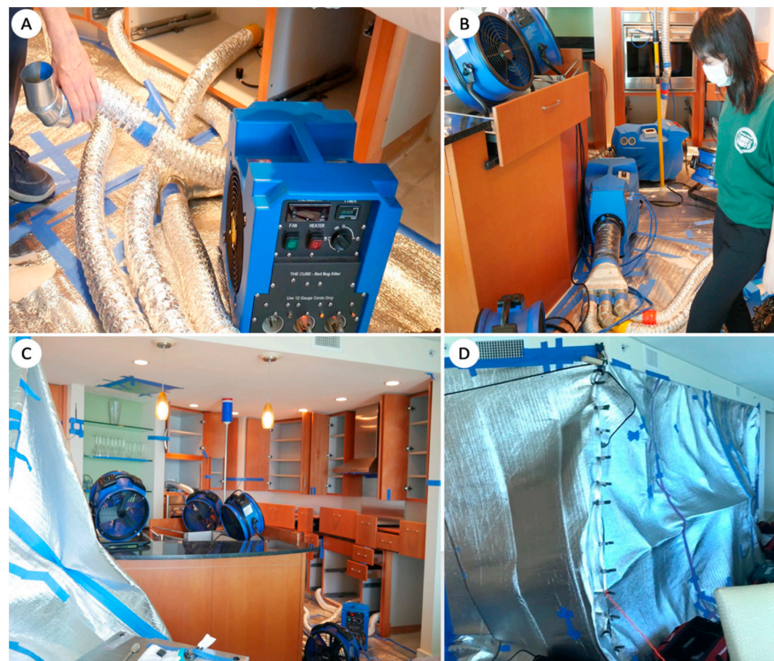
Figure 6. (A–D) Heaters (A) with distribution manifolds (B) and flexible duct pipes, and fans in place for heated air circulation (C). A treatment zone covered with a thermal blanket to contain the heated air (D).
