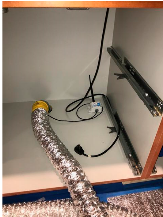
Figure 3. In each improved treatment condominium, probes ( right ) were placed in toe-kick voids for temperature monitoring and recording. Flexible duct pipes ( left ; with yellow cloth) were placed in toe-kick voids to direct heated air.
