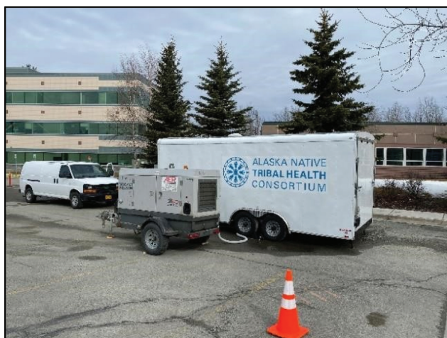
Figure 2. MST on site at Alaska native medical centre.
