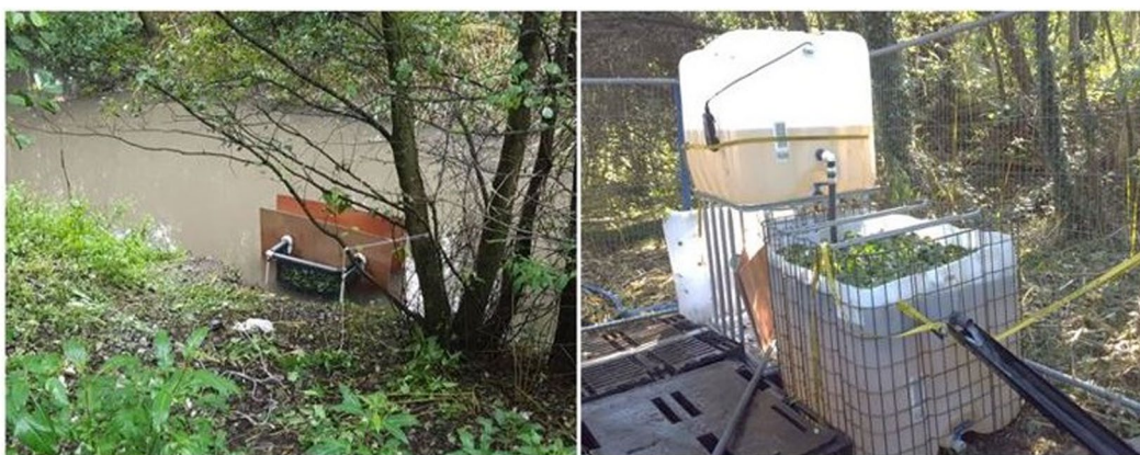
Figure 3. Photographs showing In-situ treatment pod within the Nant-Y-Fendrod (left image) and bankside treatment system (right image).
