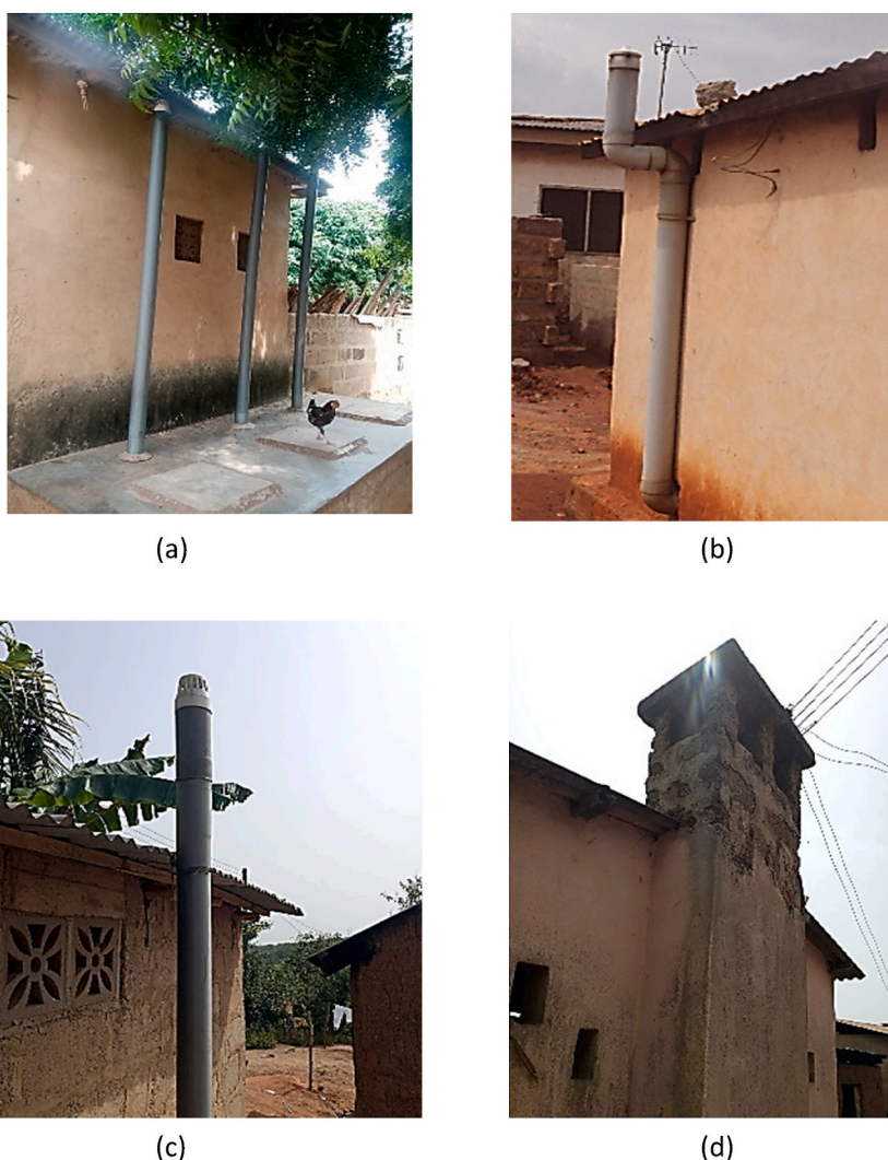
Fig. 3. Types of vent pipe materials and designs (Source: Author's fieldwork) (Note: (a) PVC pipe (75 mm diameter, below roof level); (b) PVC pipe (bent at the base and the roof level); (c) PVC pipe (installed straight and well above the roof); (d) Brickwork ventilation).
