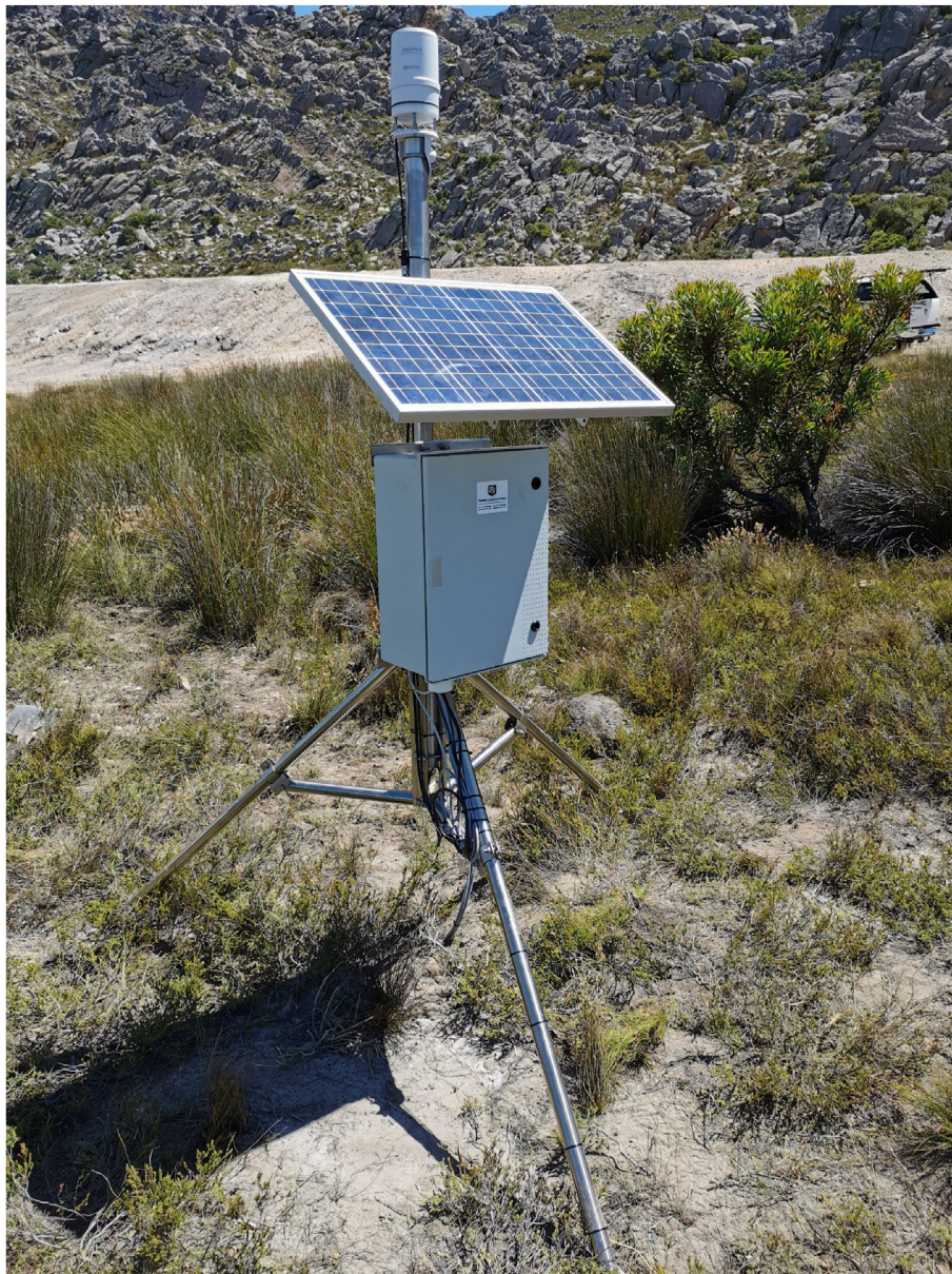
Figure 1. The climavue consisting of an integrated weather sensor at the top, a solar panel, and a cabinet containing the battery, data logger and modem.
