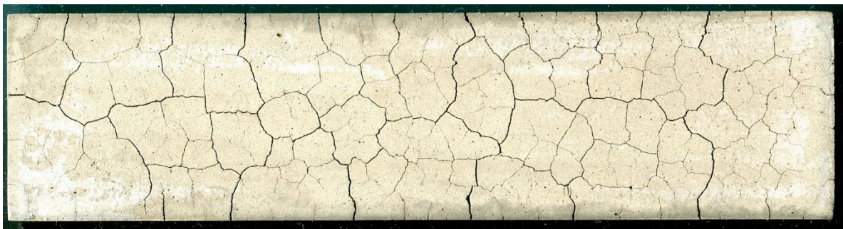
Figure 1. The cracking pattern on the surface of a cement matrix exposed to a temperature of 450 °C.
