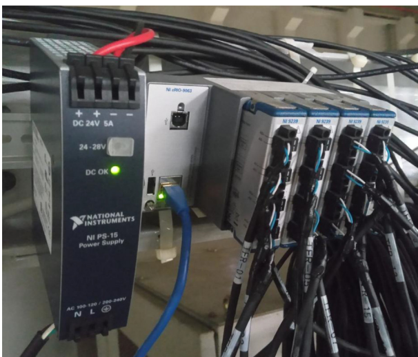
Figure 4. Picture of TFvm. Four NI 9239 modules are installed on cRIO controller.
