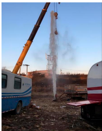
Figure 3. PF-GUN operation site. After the PF-GUN operation, the wellbore water column rushed out about 22 m due to a sudden pressure increase in the bottom hole.
