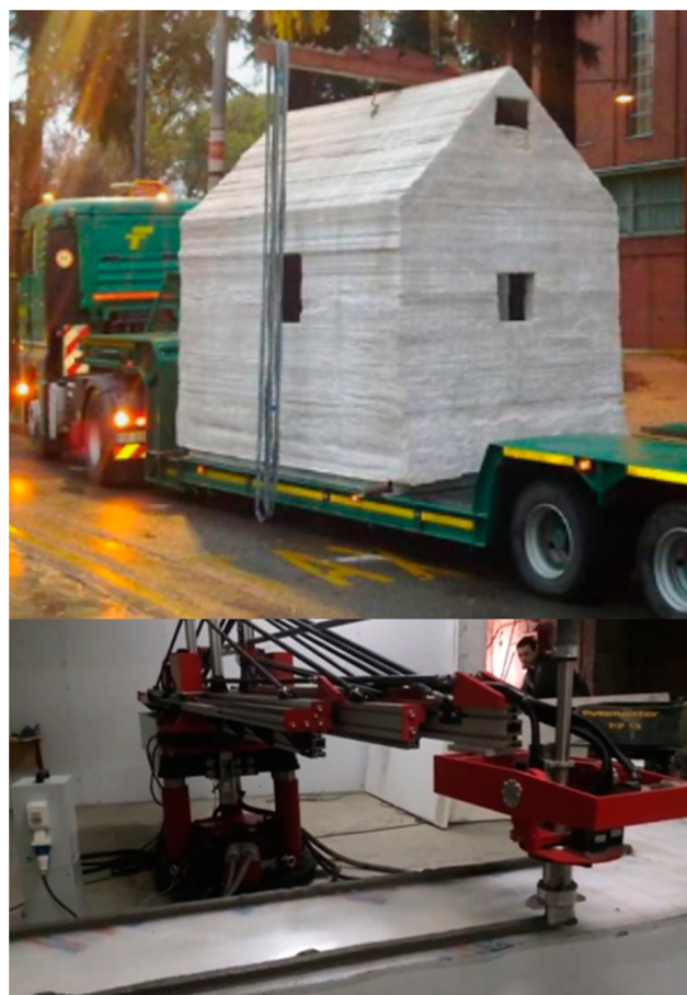
Figure 79. Top: 3D printed house fabricated via D-shape process. Image reproduced with permission from ref 810. Copyright 2014 Elsevier. Bottom: Concrete printer from Apis-Cor for on-site construction. 811 Image courtesy of www.3ders.org .
