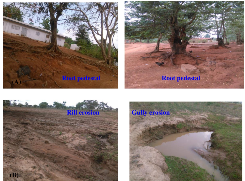
Fig 4. Indicators of erosion severity: (A) Pedestals (exposure of tree roots due to erosion in the Eastern Region), and (B) rill and gully erosion from the Northern Region as. (Source: Gebreyesus Brhane Tesfahunegn, May 2017).
