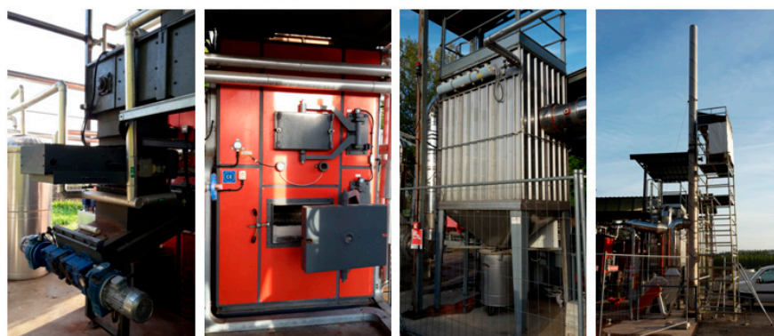
Figure 1. Details of the CHP plant (double screw mechanism, furnace, baghouse filter, and chimney).
