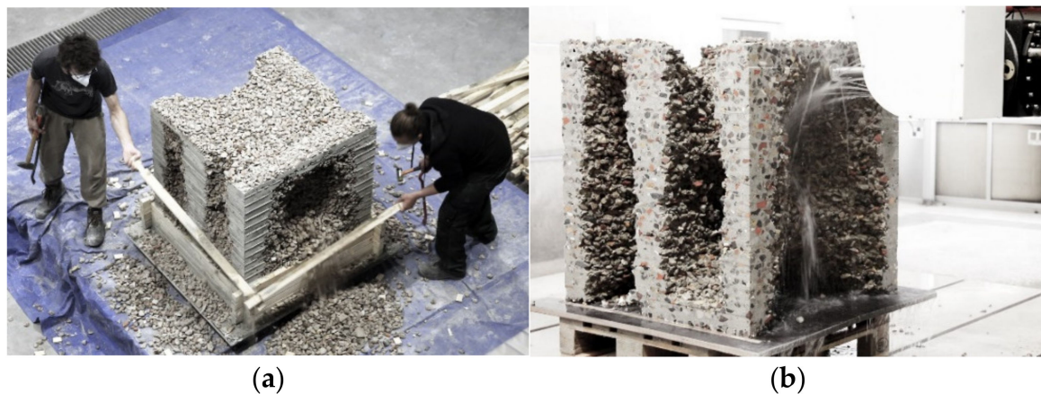
Figure 16. Demoulding and post-processing: (a) dismantling of the stackable formwork elements; (b) milling of the edges.
