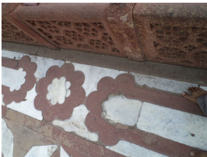
Fig. 1.16 Marble within siliceous stones damaged due to air pollutants
