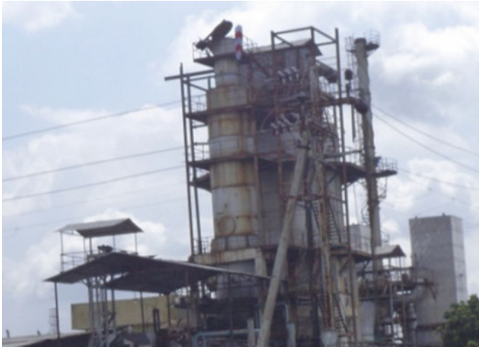
Fig. 1.21 Corroded steel structure
