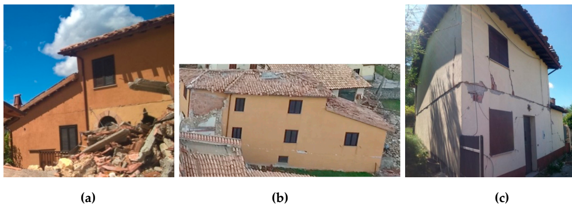
Figure 6. Crack pattern: (a,b) Building No. 2; (c) Building No. 3.
