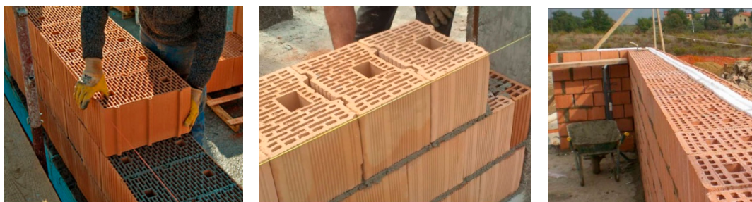
Figure 3. Construction method of hollow clay blocks: blocks are typically arranged in single-wythe walls, without mortar along the vertical joints.
