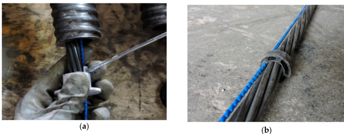
Figure 59. DOFS installation by means of plastic hooks for coupling the DOFS in an anchor's (a) extremity bar and (b) internal bar [139].
