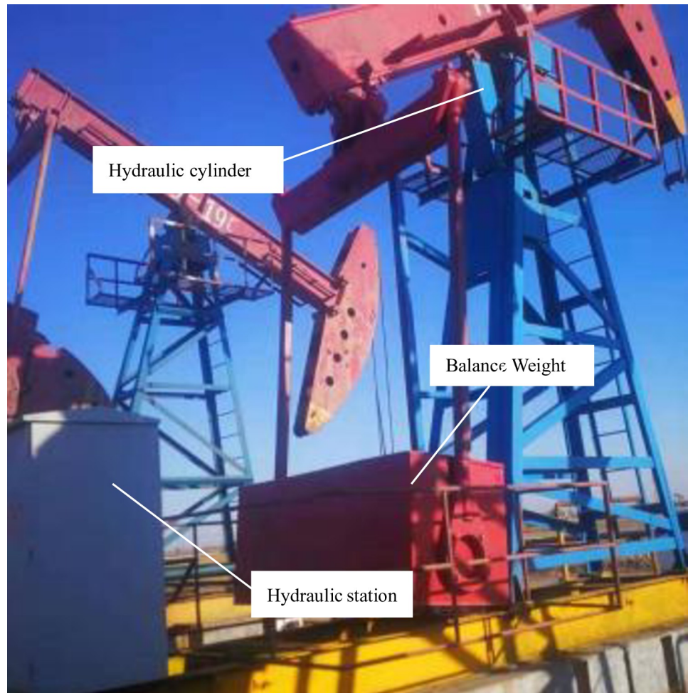
Fig 13. Hydraulic drive pumping unit.
