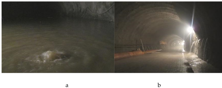
Figure 19. Photographs of water gushing from the tunnel scene: (a) normal bottom flush; (b) fracture-type normal water.
