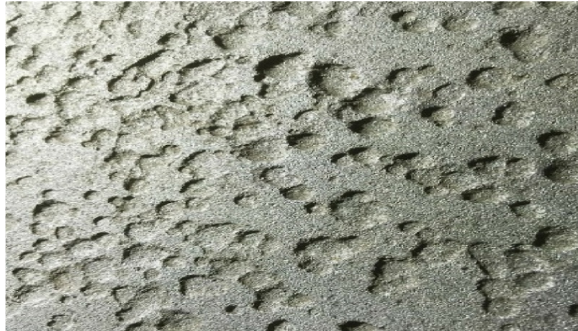
Figure 3. Example of Pitting Corrosion [12].
