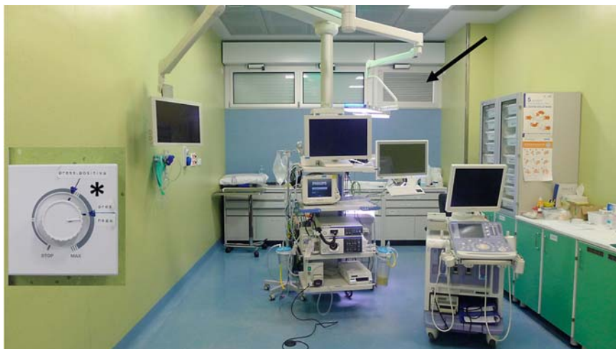
► Fig. 2 Endoscopy room with a dedicated ventilation system (black arrow) to guarantee a negative pressure (asterisk).
