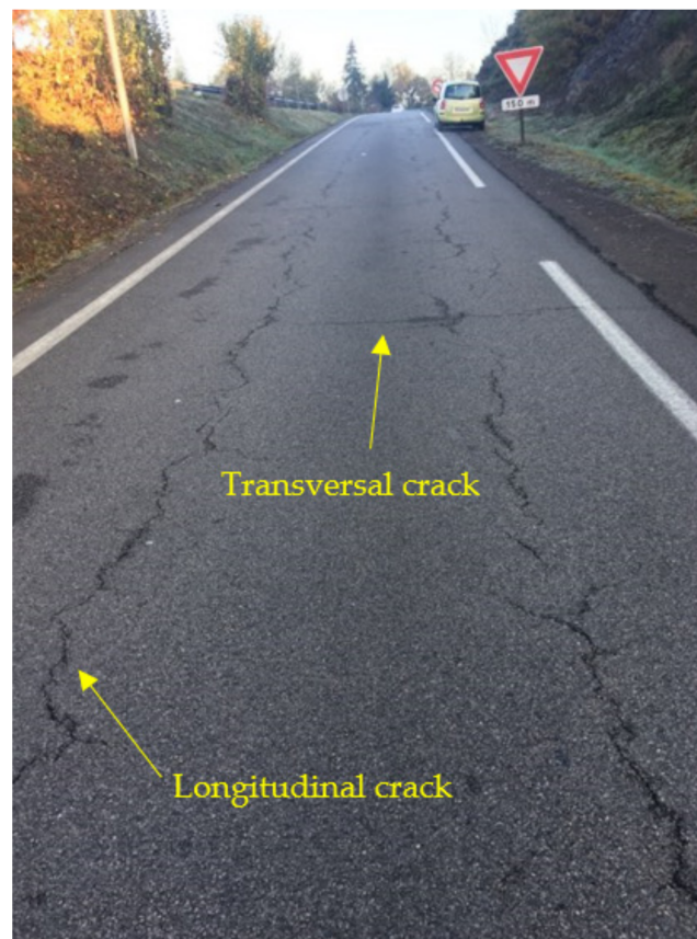
Figure 10. Cracking at the pavement surface.
