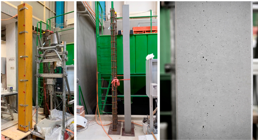
Figure 9. High-strength reinforced concrete column. From left to right: wooden formwork 150 \times 150 mm, middle reinforcement cage provided by industry partner, result of casted column.
