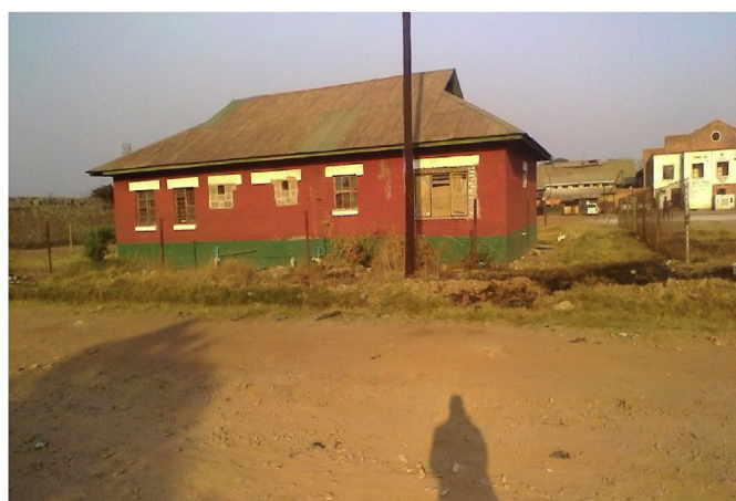
Fig. 3. Roofs and paints corroded by sulphur acidity in Kankoyo.
