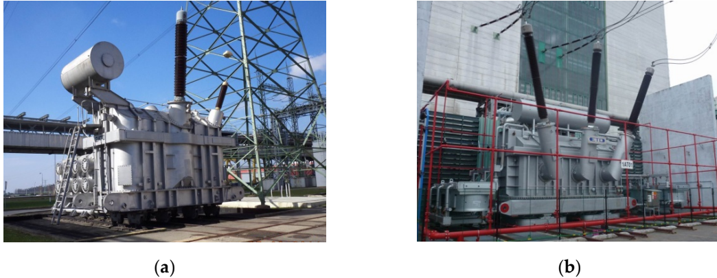
Figure 1. Examples of high-power main transformers: a single-phase 24/420 kV unit, 400 MVA (a); a three-phase 16/420 kV unit, 300 MVA (b).
