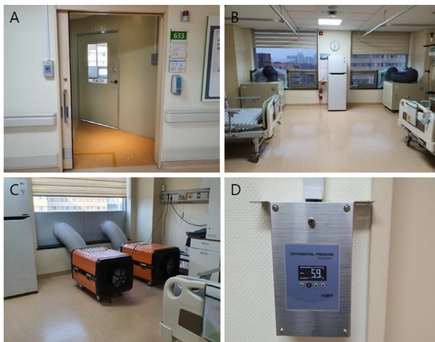
Fig 3. Examples of airborne infection isolation rooms (AIIR) and equipment installation. (A) Example of an AIIR with oblique partitioning (room 633). (B) Installation of negative air machines (model WS-H-1200, Wosem Co., Ltd., Cheongju, South Korea) with exhaust ducts connected to windows. (C) Magnified view of another type of negative air machine (model ARDC-1502, ASKO Co., Ltd., Seoul, South Korea) connected to the window and powered by wall outlets. (D) Display of the differential pressure measured by a pressure transmitter (model MDP-100, MST Co., Ltd., Seoul, South Korea).
