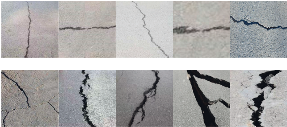
FIGURE 3: The samples of typical crack images.
