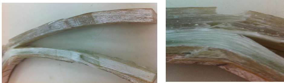
Figure 11. A severe delamination between the composite overwrapped and the joined straight pipes sections.
