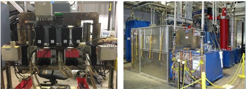
Fig. 1. H-Bridge circuit of the HVCM in the RFTF (left), high voltage and housing tank (right) connected to a klystron (red cylinder) [4].
