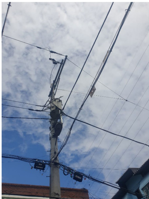
Fig. 5 Tangled electrical wires (Participant 11)
