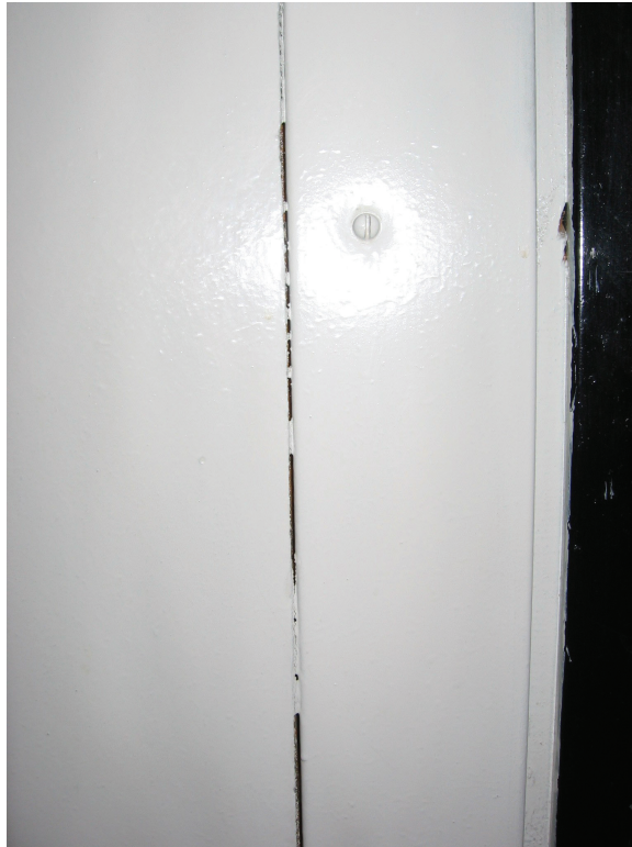
Figure 1 Example of a gap in a poorly joined CLASP column casing.
