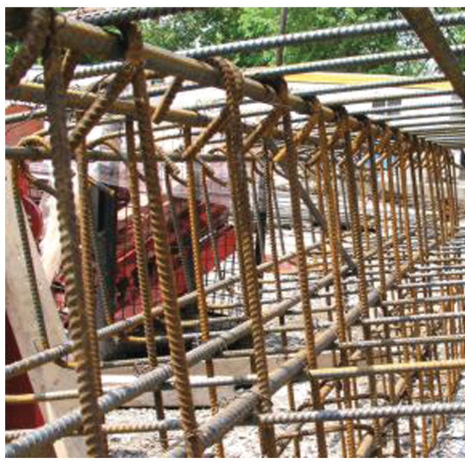
Figure 2. Steel rebar ready to be embedded in cast concrete. Note ridges on steel to help binding to concrete.
