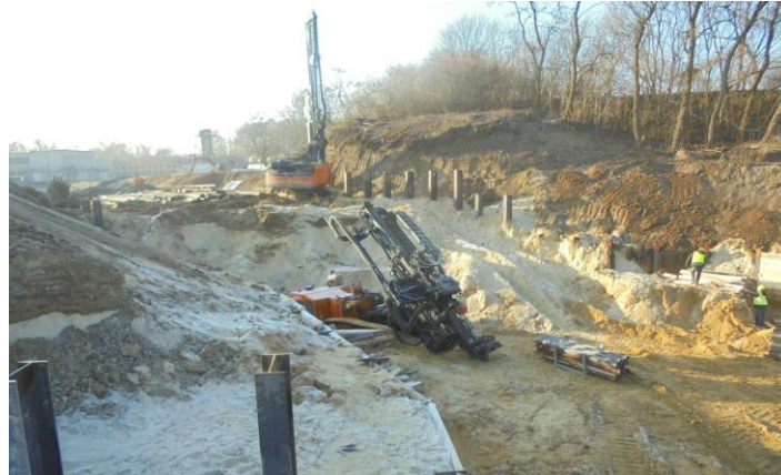
Figure 5. Passage of the communication corridor through the anthropogenic embankments: construction of the soldier pile wall. Clearly visible uncovered substrate layers of different colors.
